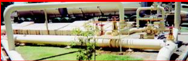
Molasses unloading facilities
