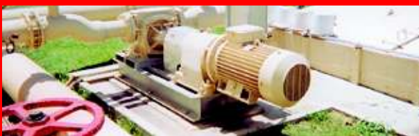
Sugar Terminal Installation
