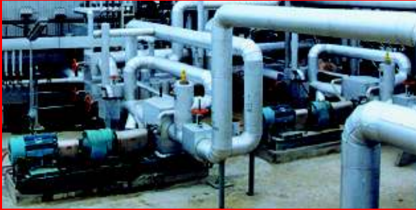
Bitumen load-out in Oil Refinery
